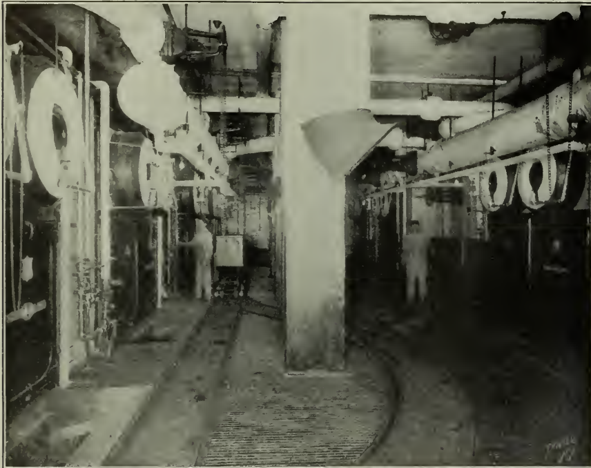
FIG. 7. FIRING FLOOR OF THE BOILER ROOM
